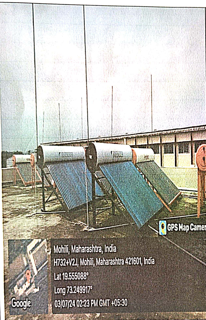
Solar Water Heater
