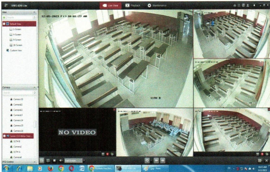
CCTV System in Class Rooms
